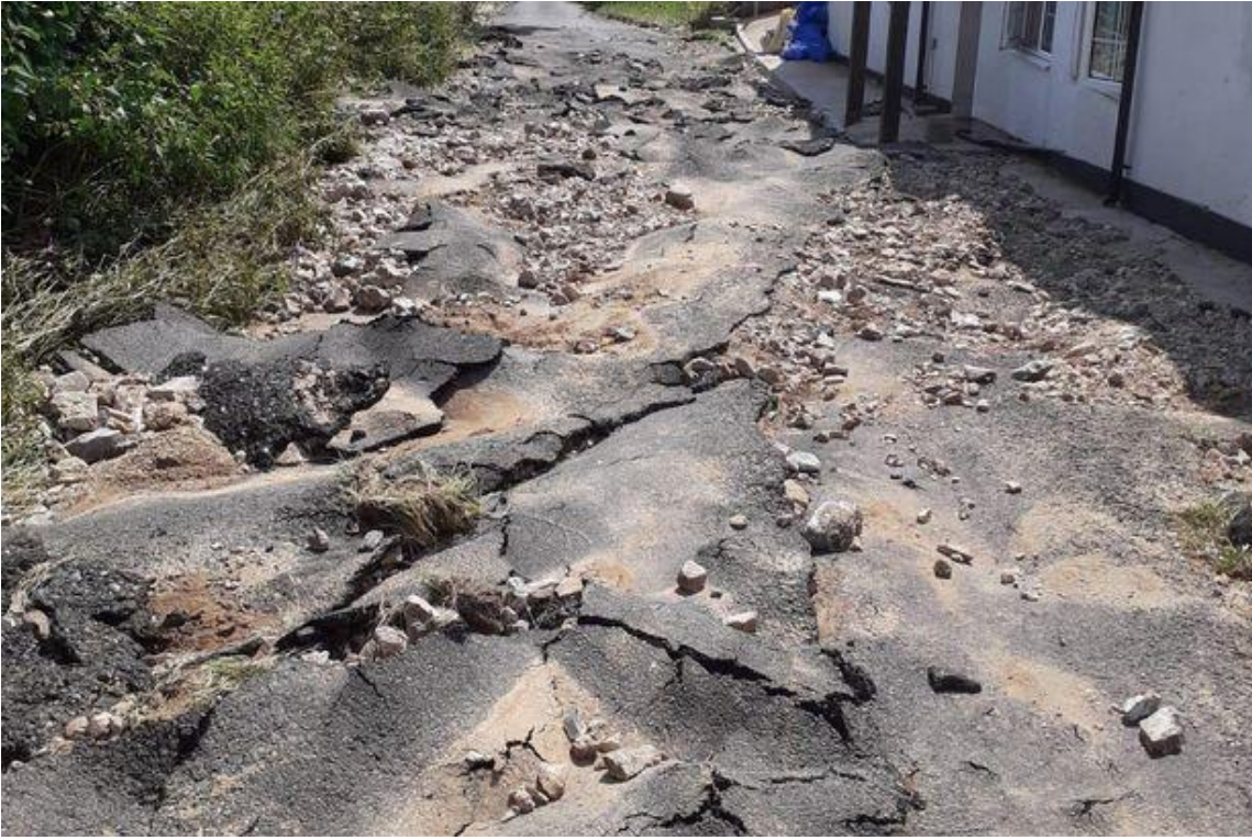
Figure 34: Damage to Scampton lane. From Chard flooding aftermath leaves roads completely destroyed - Somerset Live.
